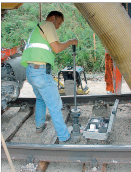
Figure 14: Establishing the resiliency modulus E_{vd} using the dynamic falling weight without disrupting progress of work
