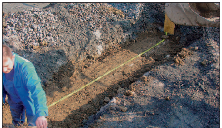
Figure 8: Lateral channels made later are the cause of localised track geometry faults which cannot be eliminated even by repeated tamping
