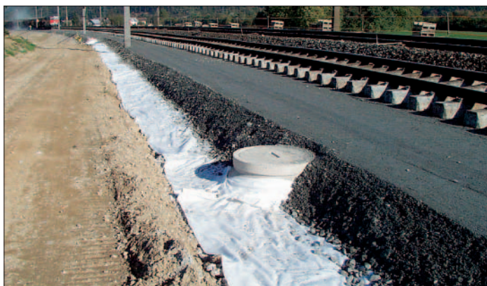
Figure 7: When the track-bed layer is integrated in the previously installed drainage system, this will increase the quality
