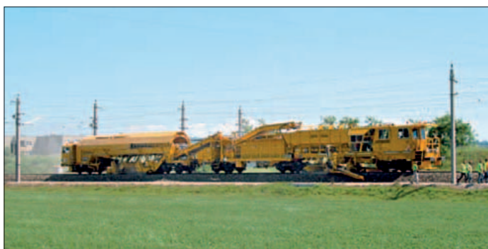
Figure 4: Machine system for ballast management
