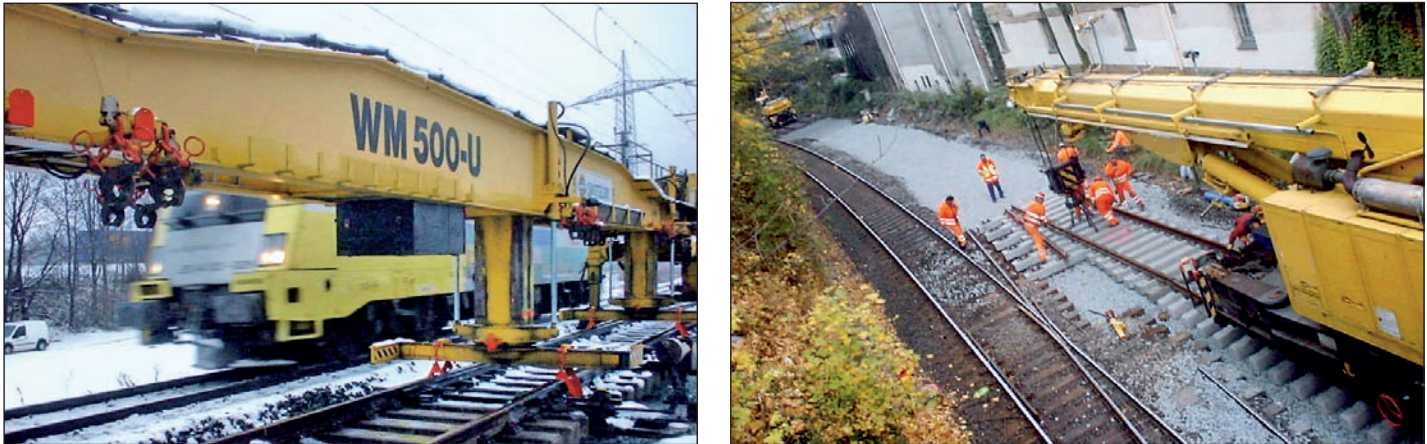
Fig. 2: Point installation using a WM 500 (left) and a railway slewing crane (right)
