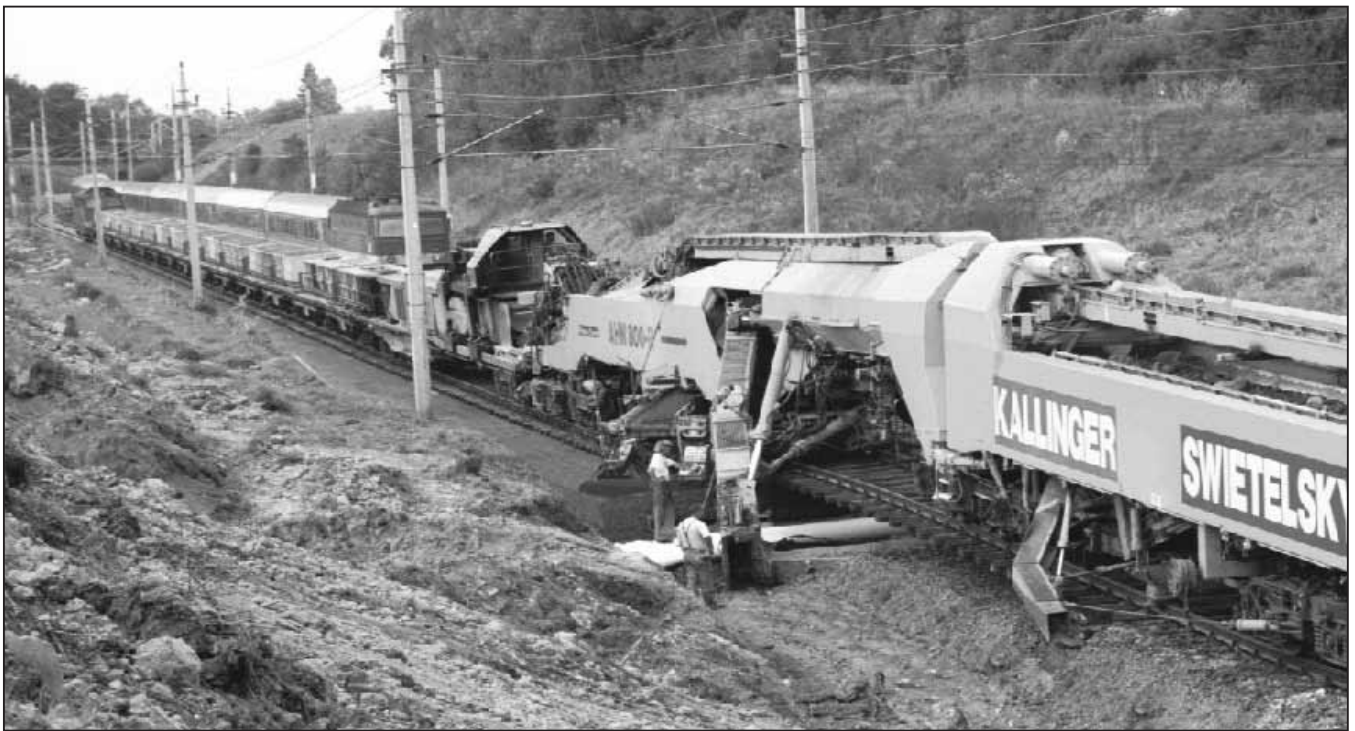
Fig. 2: The AHM 800-R formation rehabilitation machine during operation on the line Vöcklabruck - Attnang Puchheim, Track 1
