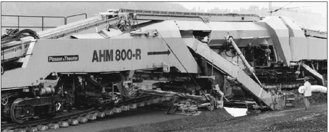
Fig. 11: Strengthening of the formation, using the AHM 800-R (line Timelkam - Redl Zipf)
