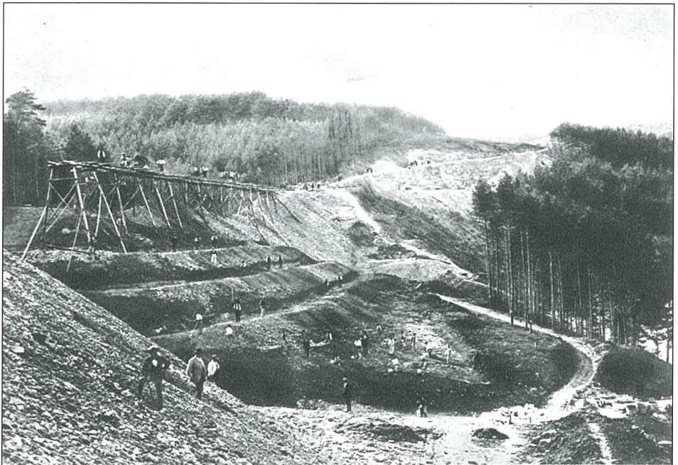
Above: Fig. 7: Scaffold construction of an embankment on the Weimar to Gera line around 1875.
