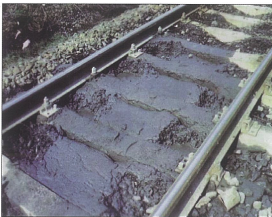
Fig. 1: Loss of load-bearing capacity in the track at a wet bed.
