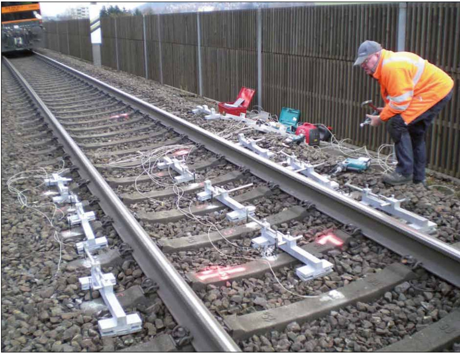
Fig. 9: Measurement setup to determine the relative vertical sleeper subsidence (Manufacturer of measurement equipment: PJM)
