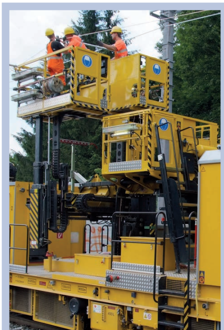
Fig. 13: Safety at the top – MTW 100.216 (symbolic photo)
